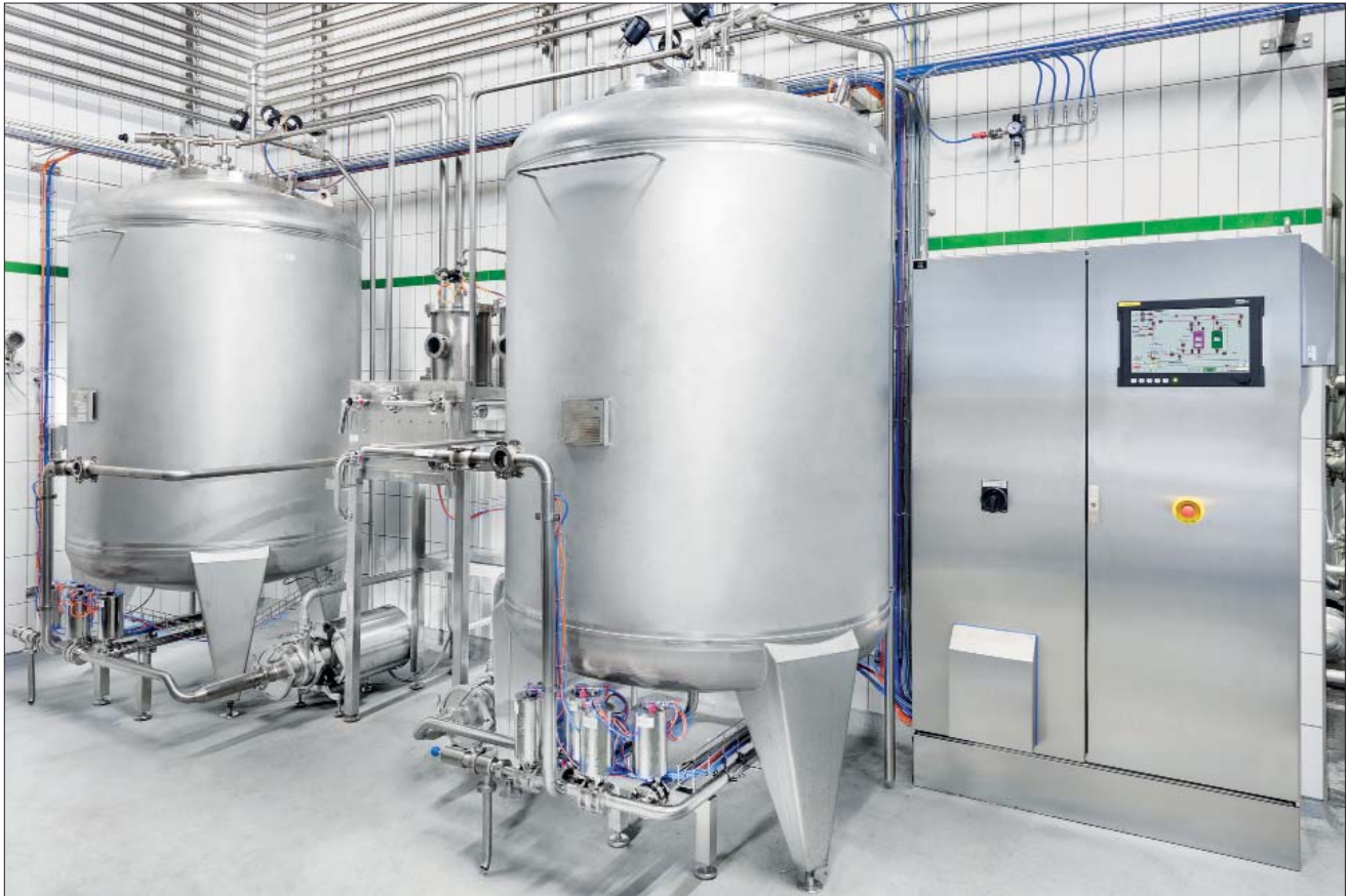
CONTI FLASH pasteurisation with a capacity of 50 hl/h
